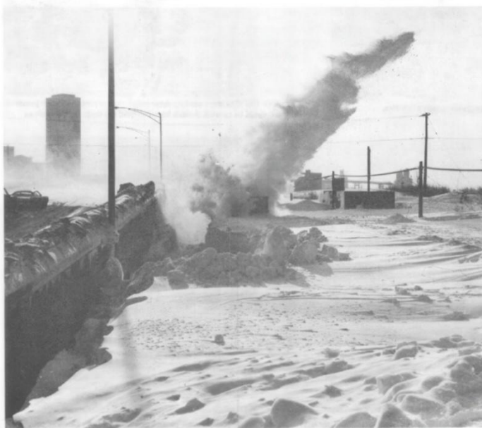
JET STREAM of snow is blasted clear of track by rotary plow at a Buffalo yard. (Fred Furminger photo)
